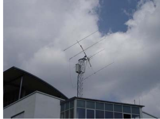
Fig. 9: Ground station antenna mounted on top of the Computer Science Department
